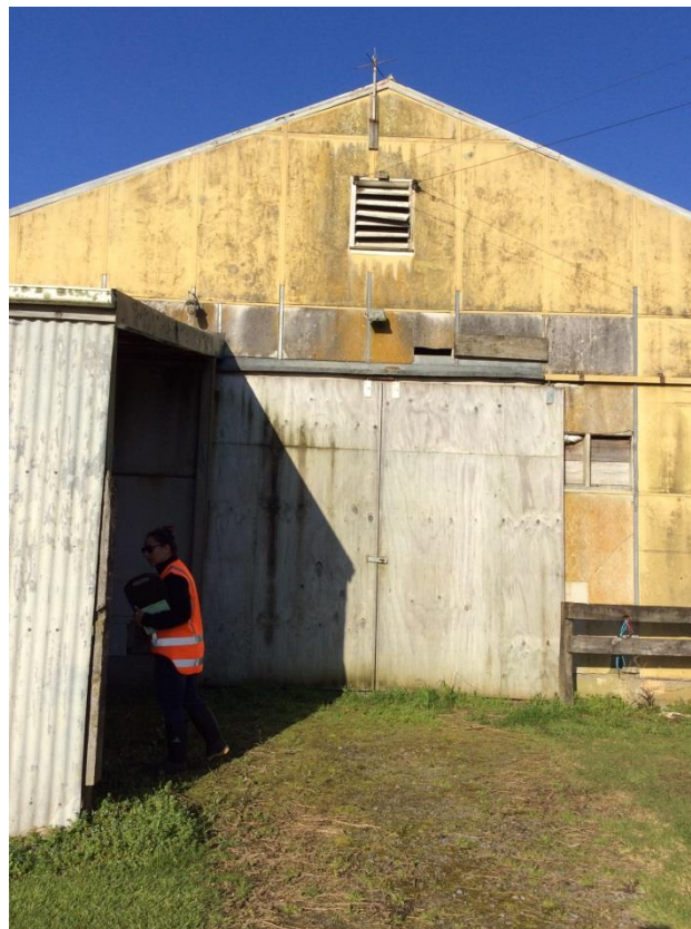
Photograph 2: Barn located on site showing ACM in deteriorated condition.
