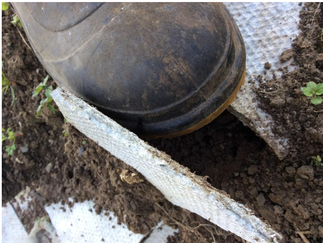
Photograph 3: Fibre cement board cladding in deteriorated condition from the barn, identified as ACM.
